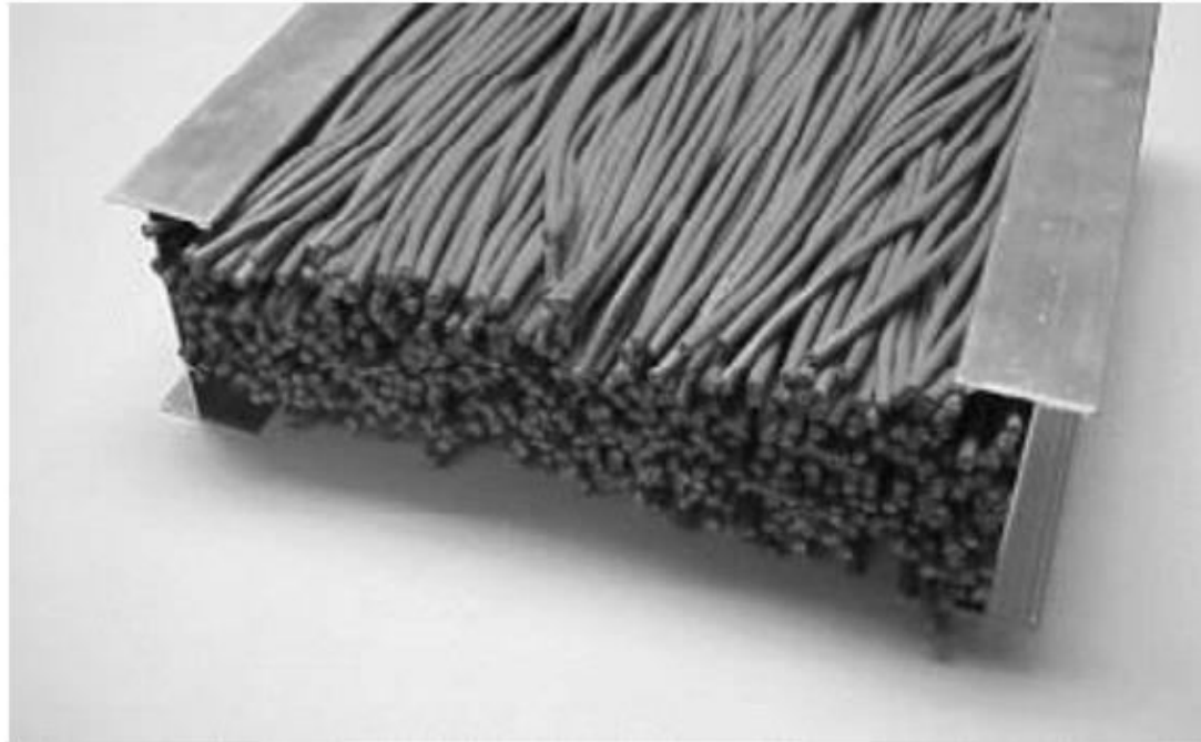
Figure 14 Cable tray with 5.5 mm (0.22 in) diameter cables at 50% calculated fill
